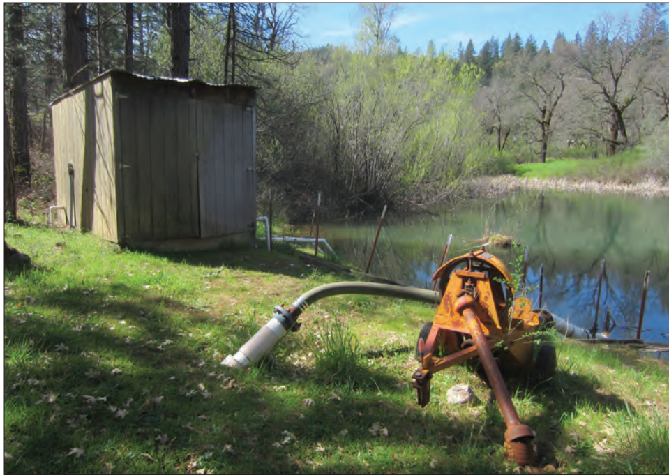
Photo 7 View of pump house at the lower pond in the western portion of the project site, looking southwest.
